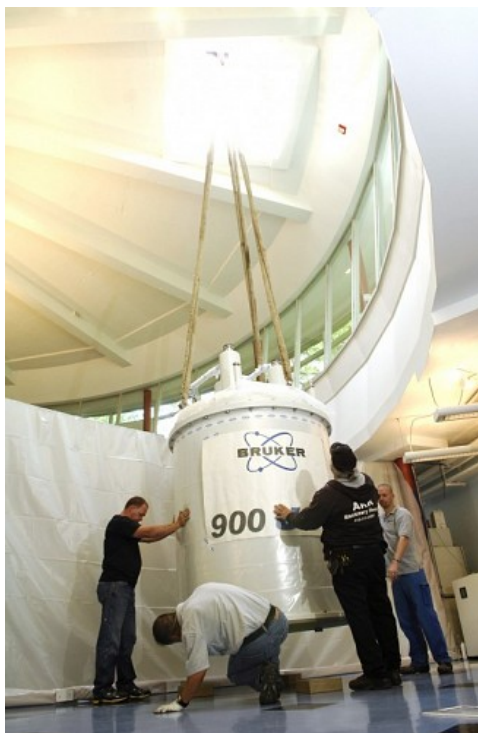
Workers install the new 7.5-ton magnet in the Biomolecular Nuclear Magnetic Resonance Facility. The magnet is part of an ultra-high field NMR spectrometer that will be among the most powerful in the nation. (photo by Anne Rayner)
